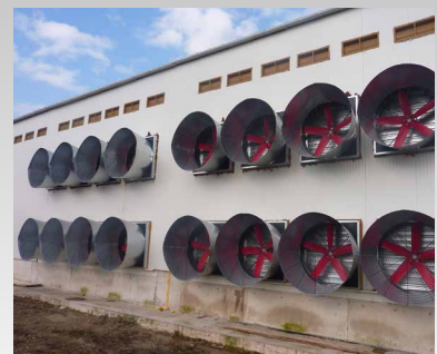
Galvanized Cone Fan in poultry house
