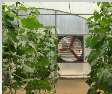
Galvanized Box Fan in greenhouse
